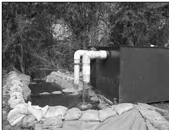
Dewatering Tank (Source: http://www.dot.ca.gov )
